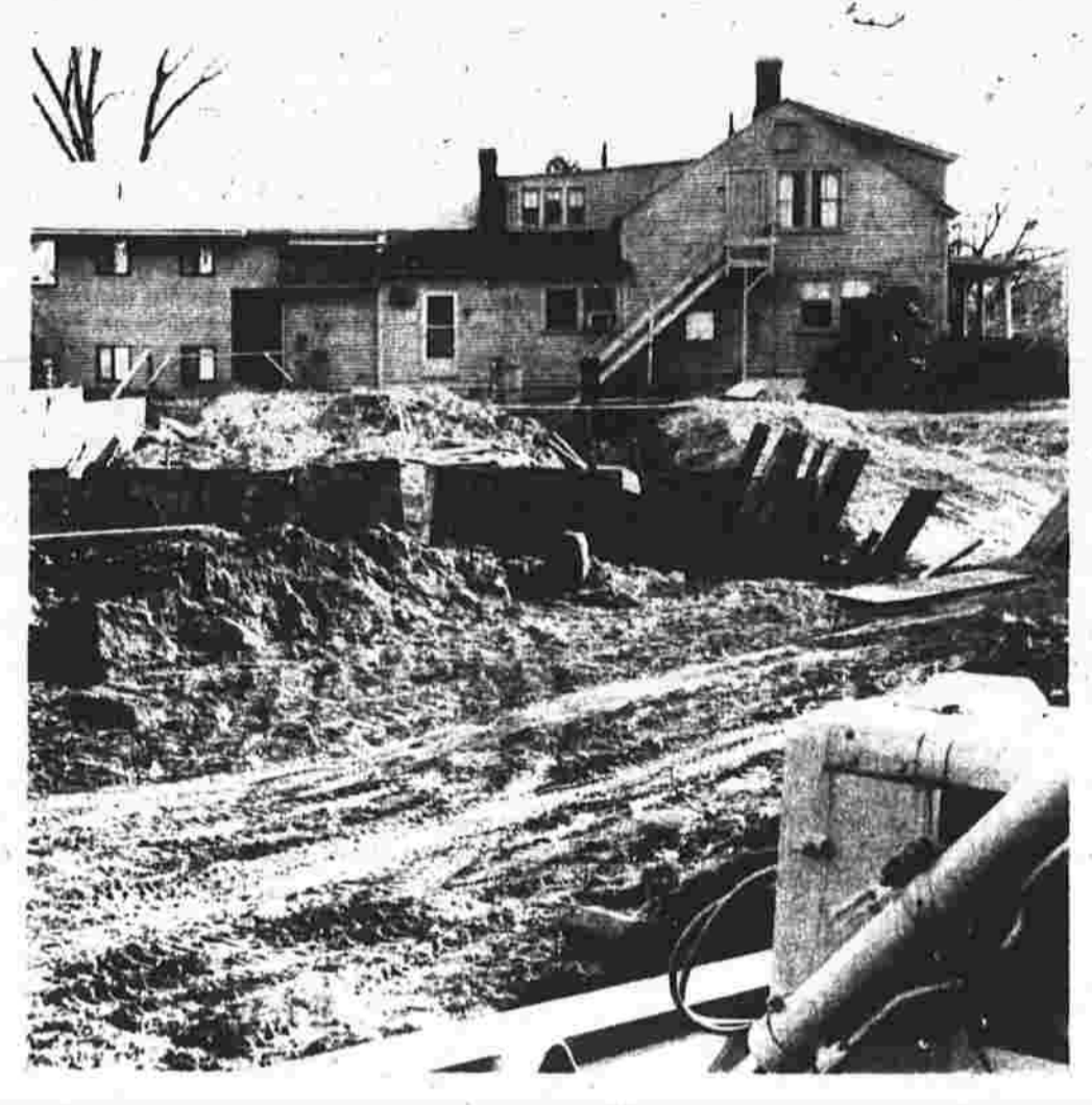
Construction is under way at the Child Guidance Center where a new wing is being built which will be joined to the one now built. At the right is the house built in 1827 being built. (Herald photo by Pinto)
